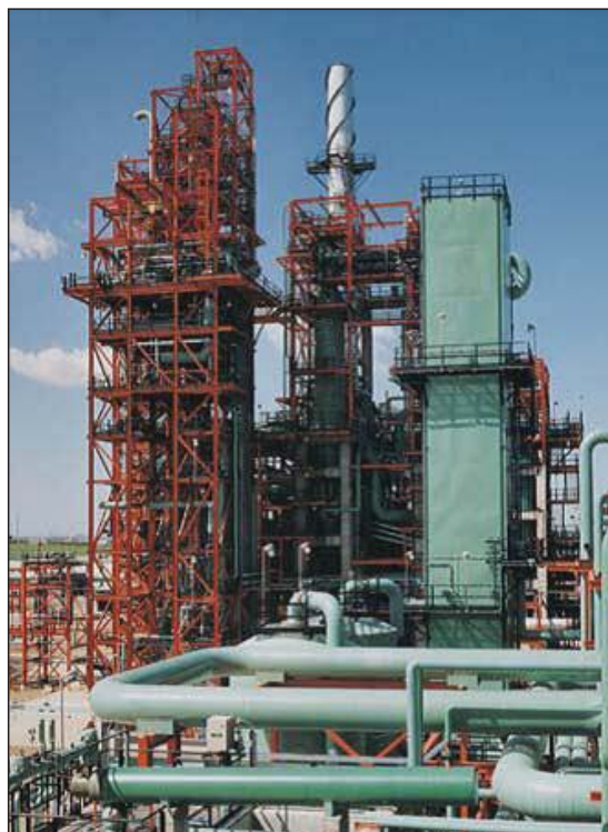
Fig. 10. The UOP Oleflex™ Process produces polymer grade propylene from a propane feedstock (Photo courtesy of UOP, A Honeywell Company)
