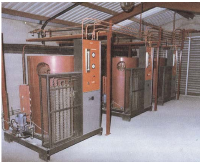
Fig. 4 The G30 (Mark II) hydrogen generator installation at the E. I. Company Ltd., Shannon, Eire. The three G10 modules each show their vertical heat exchangers mounted behind a metal grid and small gas control panel. The units are housed in a building with louvered walls, visible here at the far end. The hydrogen is used in the manufacture of electronic products and for the production of television tubes. This was the most economic and reliable solution to the hydrogen requirements of E.I.
