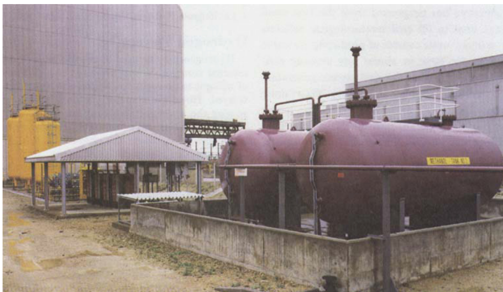
Fig. 5 A G40 (Mark I) generator installed at the Central Electricity Generating Board power station, Isle of Grain, Kent. The Dutch Barn shelter provides adequate protection for the four G10 modules. In the foreground are the methanol tanks which hold six months' supply of fuel. The yellow vertical pressure vessels are for storing hydrogen which is used for cooling the alternators. This application is a major outlet for methanol-fuelled hydrogen generators; the self-sufficiency they provide to remote power stations has already proved to be of especial value
