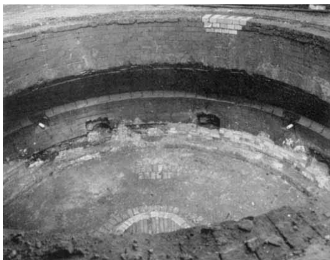
A circular soaking pit at the Ebbw Vale works of Richard Thomas and Baldwins Limited. Two of the four control thermocouples can be seen projecting from the wall
