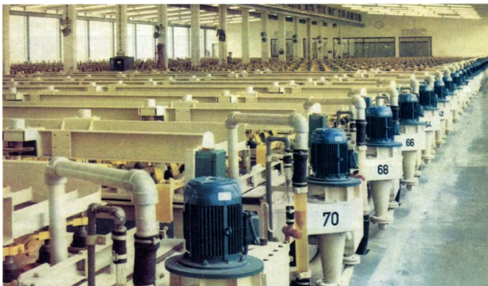
Fig. 5 The vast size and apparent inactivity of a mercury-type chlorine cell room belies the complexity of construction and continuous high current density electrochemical reactions in progress. This cell room will contain many thousands of titanium-based electrodes
