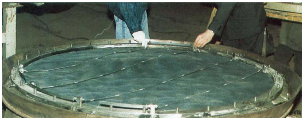
Fig. 2 A view of the four parallel heating elements of an electrical ignition device installed in a UKL-7 ammonia oxidation reactor. The elements are ~ 500 mm apart. The UKL-7 is a Russian-designed non-concentrated nitric acid plant and this particular one belongs to JSC 'Achema' in Jonava, Lithuania
